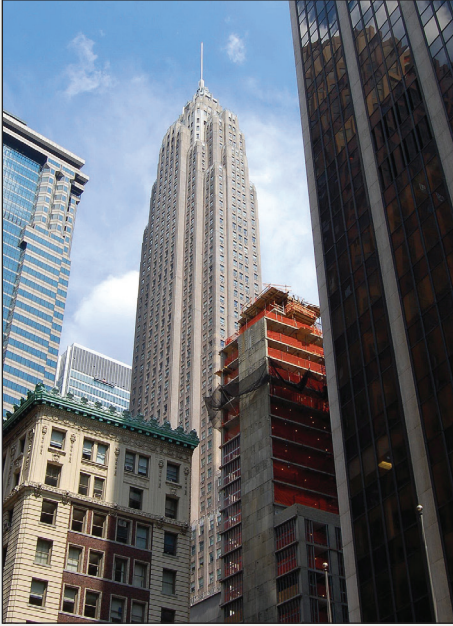
70 Pine Street New York, NY Developer: Rose Associates Architect: Stephen B. Jacobs
